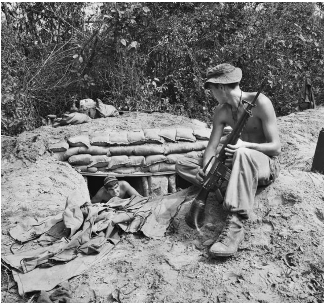
An infantryman from 3RAR, watched by another, makes repairs on his bunker after it was struck by mortar fire during a North Vietnamese attack on Balmoral
